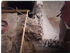
The original gutter was redone, as was the area around the column.
